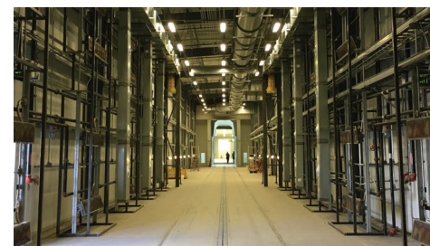
Oven with IR Heaters in place
